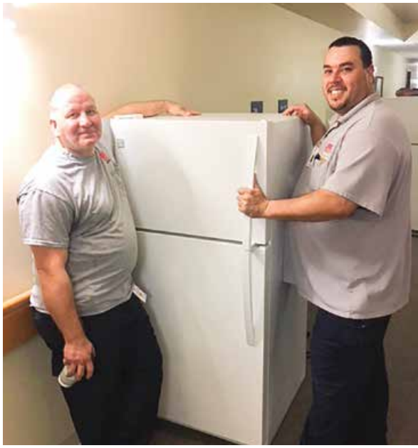
HDC MidAtlantic Maintenance Technicians Rod Ashman (left) and Nayip "Junior" Segerra assist with the installation of the energy efficient refrigerators at Penns Common Court in Reading, Pa.
